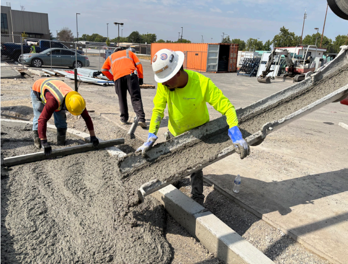
Total Site Services pouring the curbs outside the sallyport in prep for asphalt.
